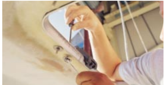
The hatch should be through bolted in the hinge areas, while self-tapping screws can be used for fitting the remainder of the lower frame to the deck sheet.
